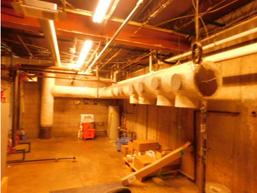
View of basement utility room, with asbestos containing TSI coated heating system pipes. The piping appears to be inactive and disconnected.
