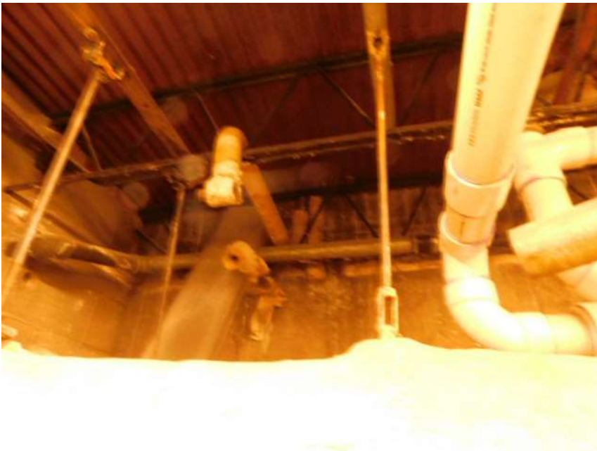
View of small diameter insulated water line piping above the large diameter TSI coated piping.
