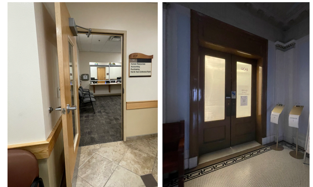
Doors need to be held open for wheelchair users.
